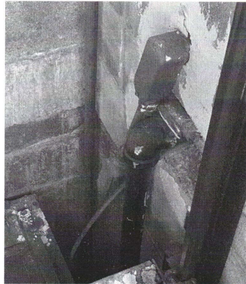
14. South - Hoistway penetrations should be properly sealed.
