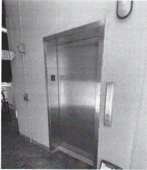
41. North – Corridor button fixtures to be replaced with vandal-resistant fixtures.
