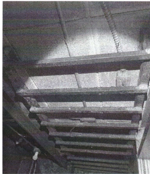
22. South – New code compliant pit access ladder should be installed.
