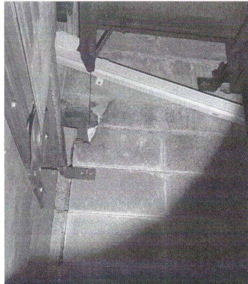
24. Damaged block in the elevator hoistway must be repaired.
