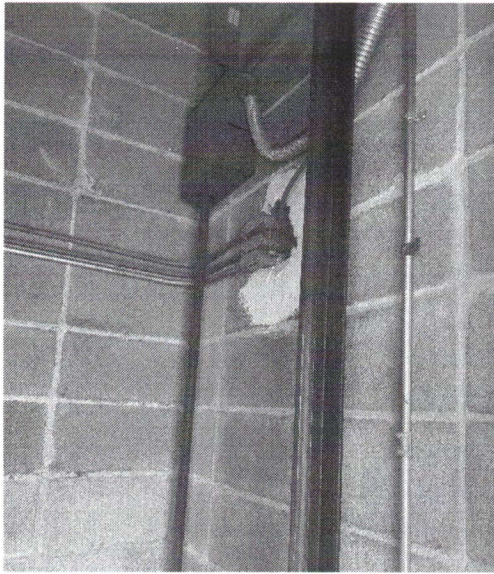
17. South - Hoistway penetrations should be properly sealed.
