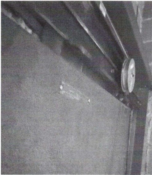
19. South – New hoistway door tracks and hangers should be replaced due to rusted condition.
