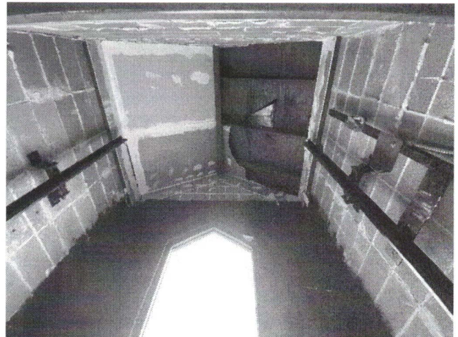
40. North – Sheetrock at top of elevator hoistway must be repaired for proper fire rating.
