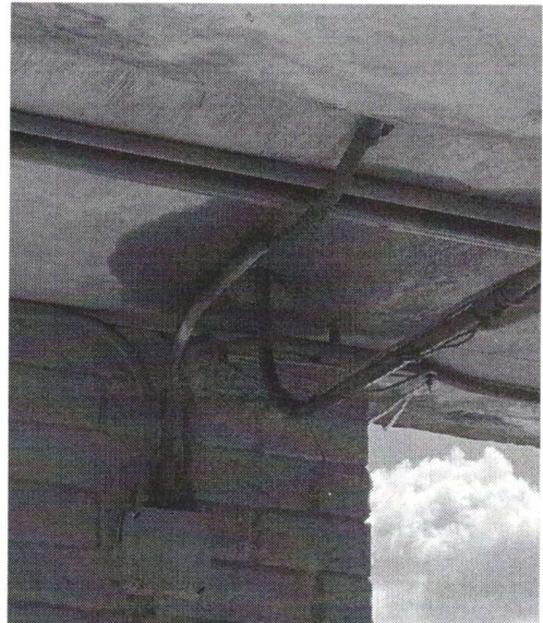
42. North – Leaking power unit is penetrating through the machine room floor onto the building overhead on the "G" level.
