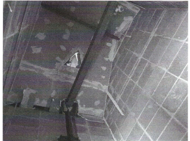
18. South – Sheetrock at top of hoistway should be properly repaired.
