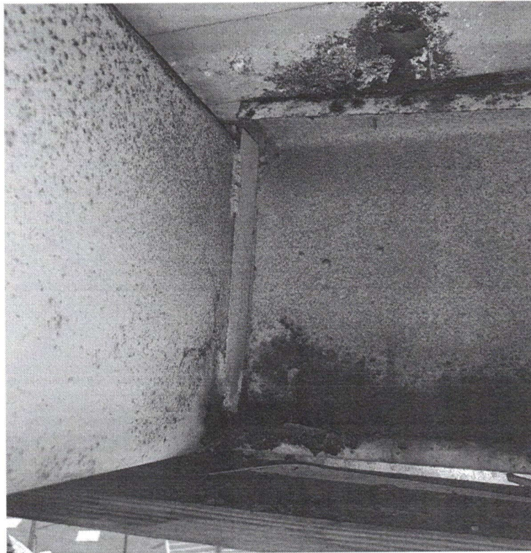
Photo No. 26 – Deteriorated Rim Joist to be Replaced
